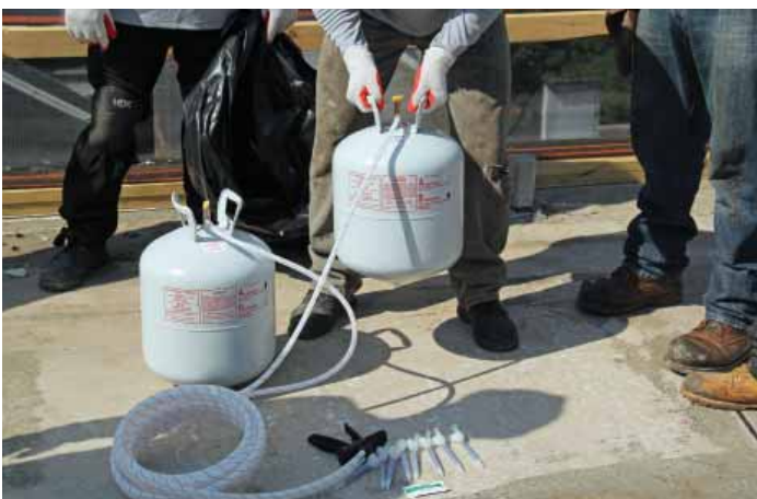
Shaking of A-side and B-side tanks
